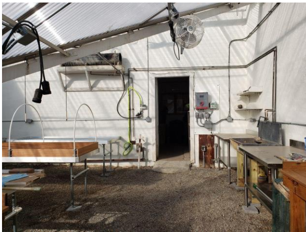
New Electric Panel for vent operations
